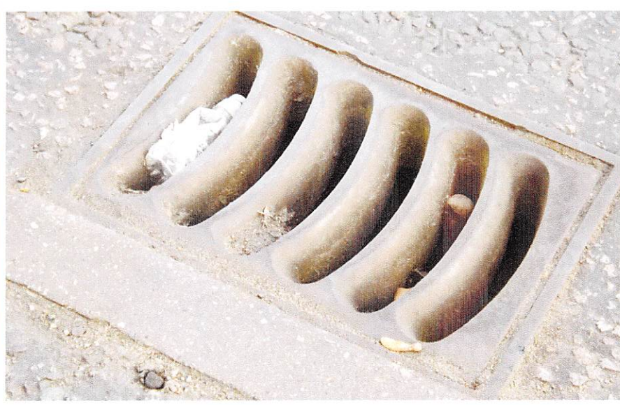
Fig.13 Drains getting blocked by litter.
